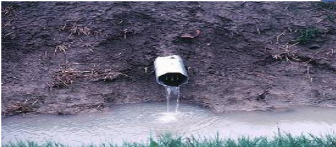
Drain tile outlet to a drainage ditch
