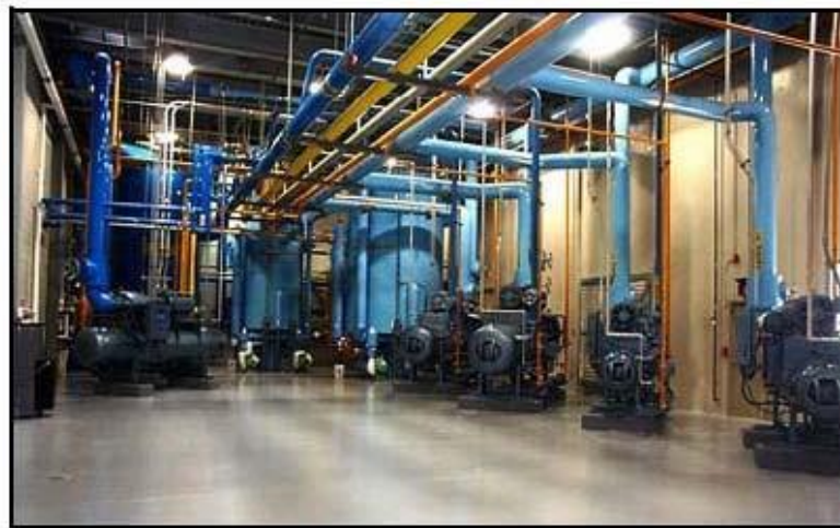
Fig.3.2. Ammonia based refrigeration plant for a large cold storage
