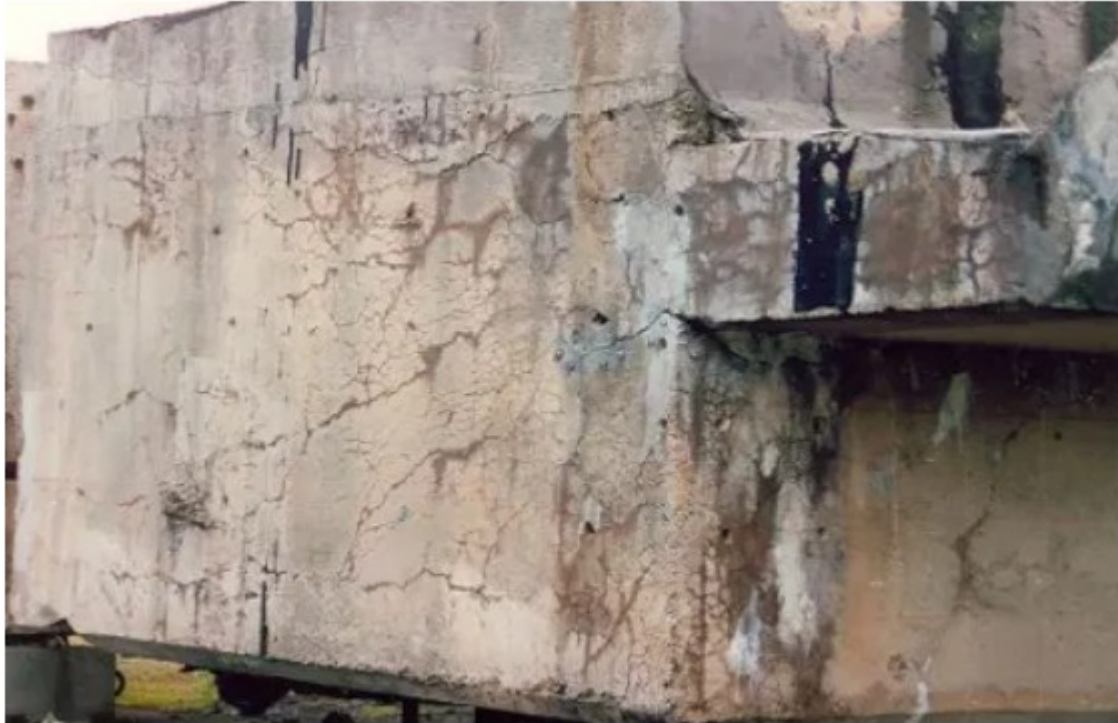
Fig 8: Effect of Alkali Aggregate Reaction on Concrete
