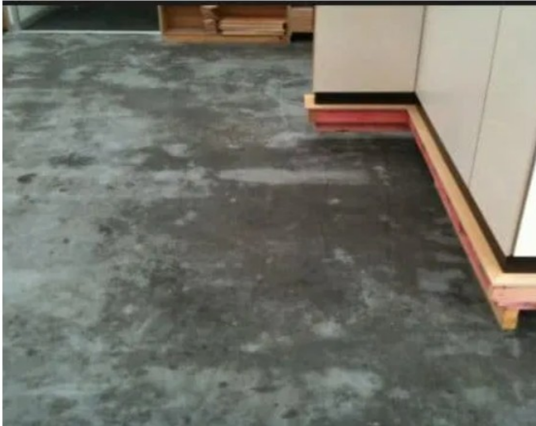
Fig 6: Dampness on Concrete Surface
