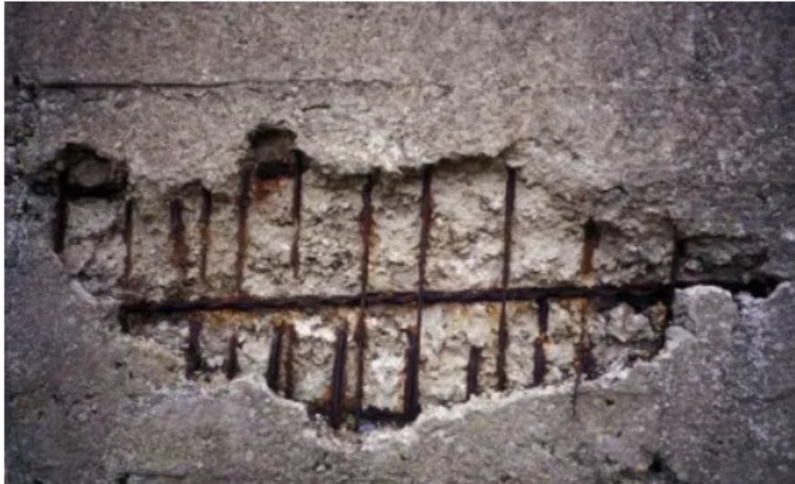
Fig 11: Corrosion of Steel in Concrete
