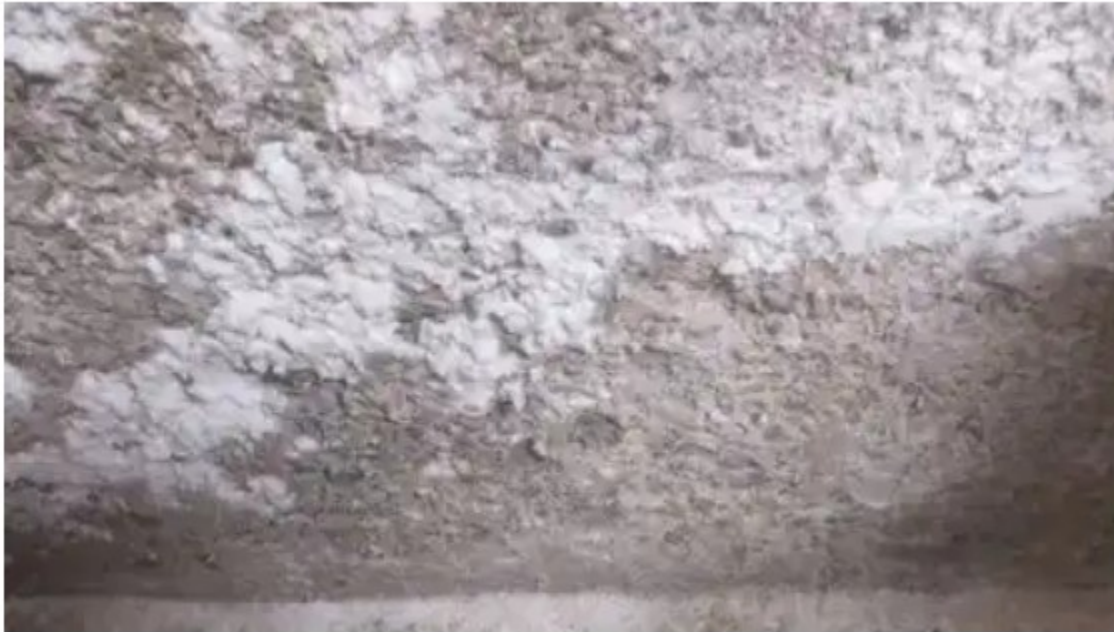
Fig 13: Concrete affected by Fungi
