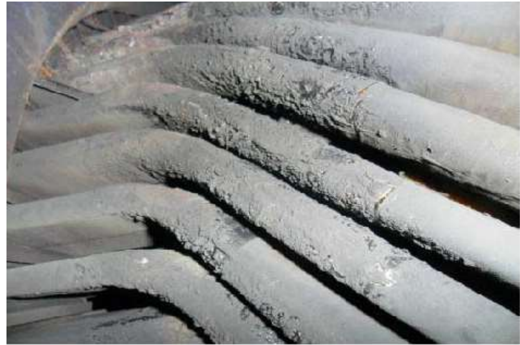
1. Stator windings burned by oil-contamination discharge.
