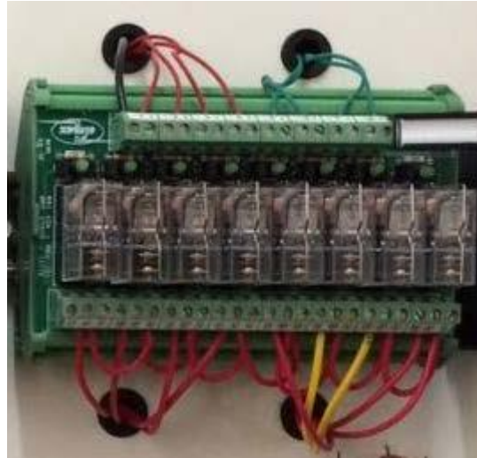
Fig Relay Unit.
