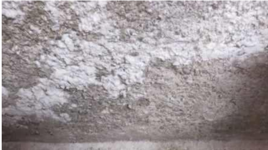
Fig 13: Concrete affected by Fungi
