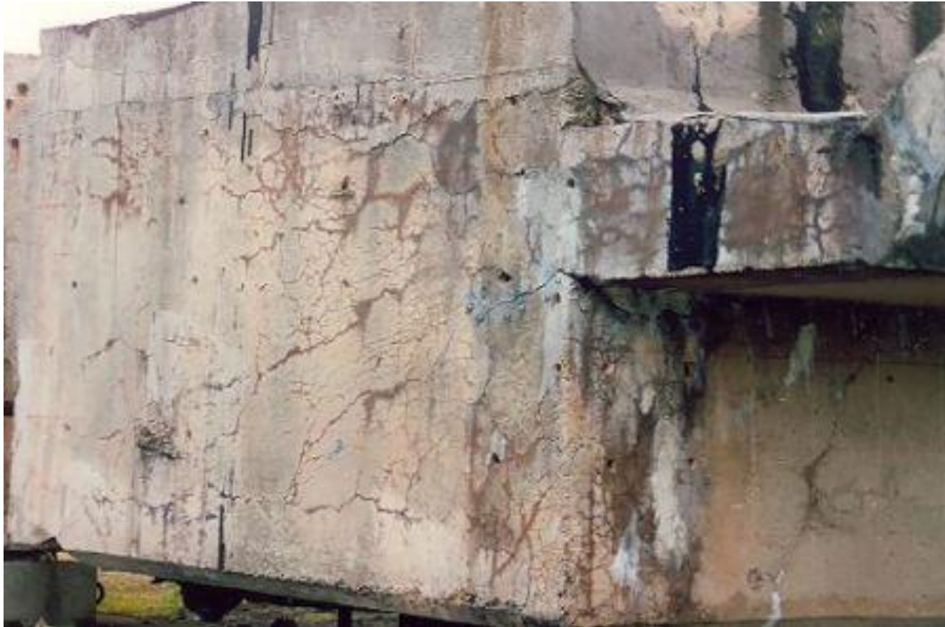
Fig 8: Effect of Alkali Aggregate Reaction on Concrete
