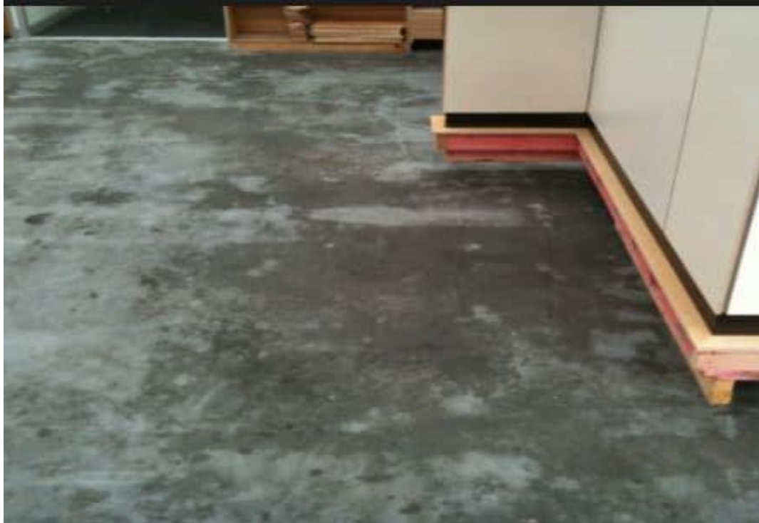
Fig 6: Dampness on Concrete Surface
