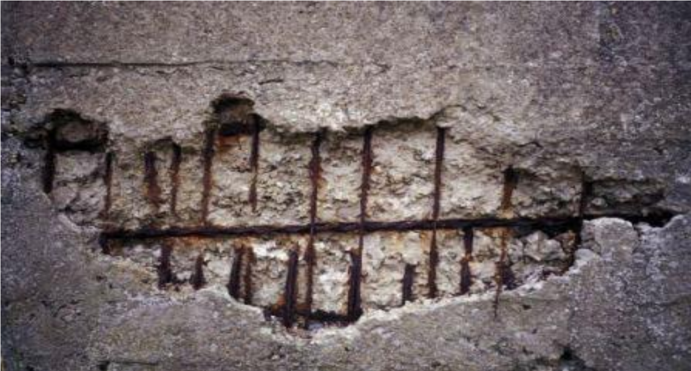
Fig 11: Corrosion of Steel in Concrete
