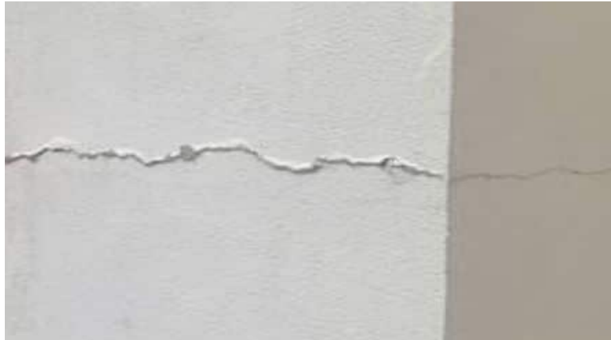
Fig.2: Cracking due to thermal movement
