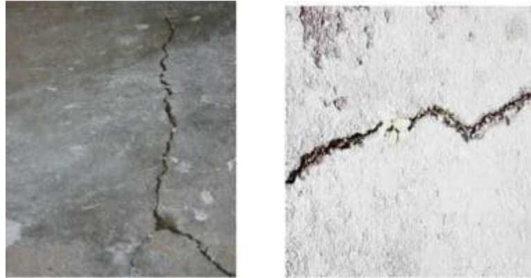
Fig.9:Concrete building cracking due to poor construction practice; water added to fresh concrete
