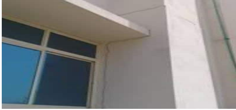
Fig.7:Crack above window due shrinkage
