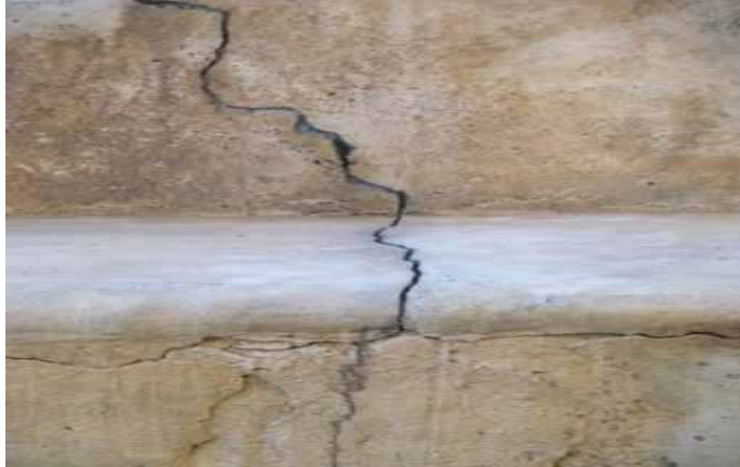
Fig.4:concrete building cracks due to creep movement
