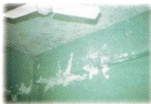
Fig.11:Leakage from roof slab
