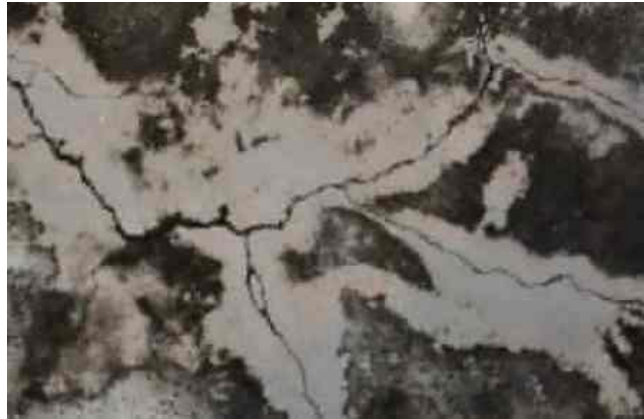
Fig.8:concrete cracking due to moisture movement
