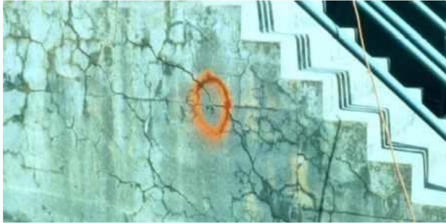
Fig.12:Cracking due to alkali-silica reactions
